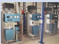
the MULTIPLE STEAM GENERATING UNIT MDA
